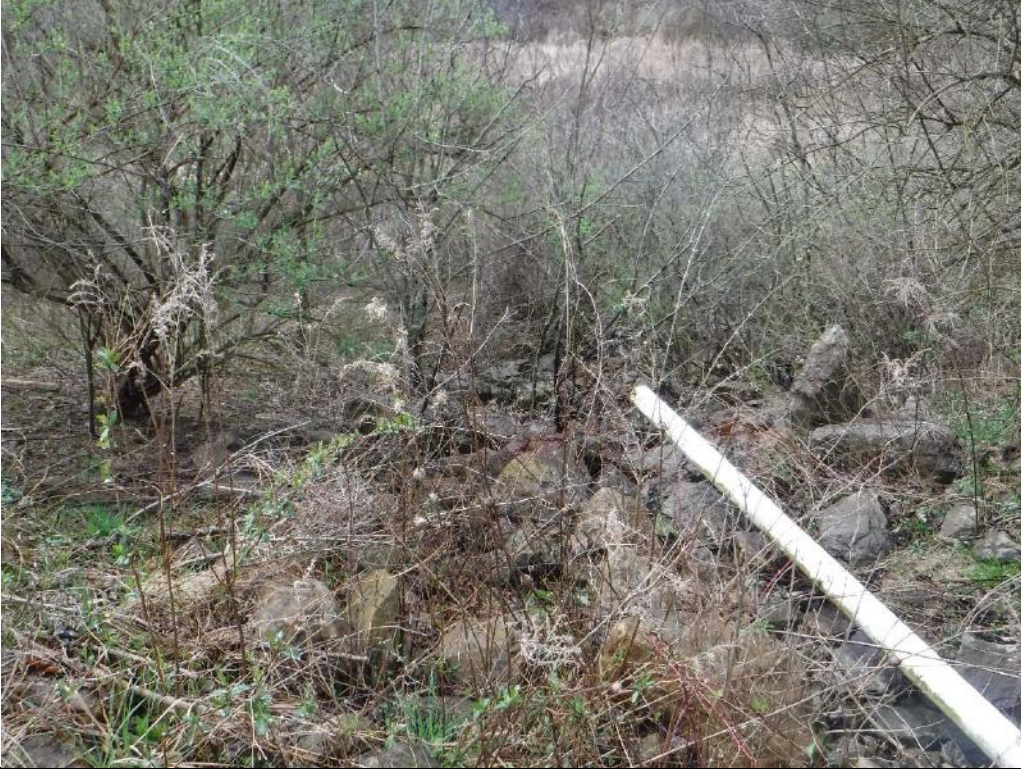
Photograph #21 | Outfall pipe located at convergence of drainage swale, southernmost portion of site.
